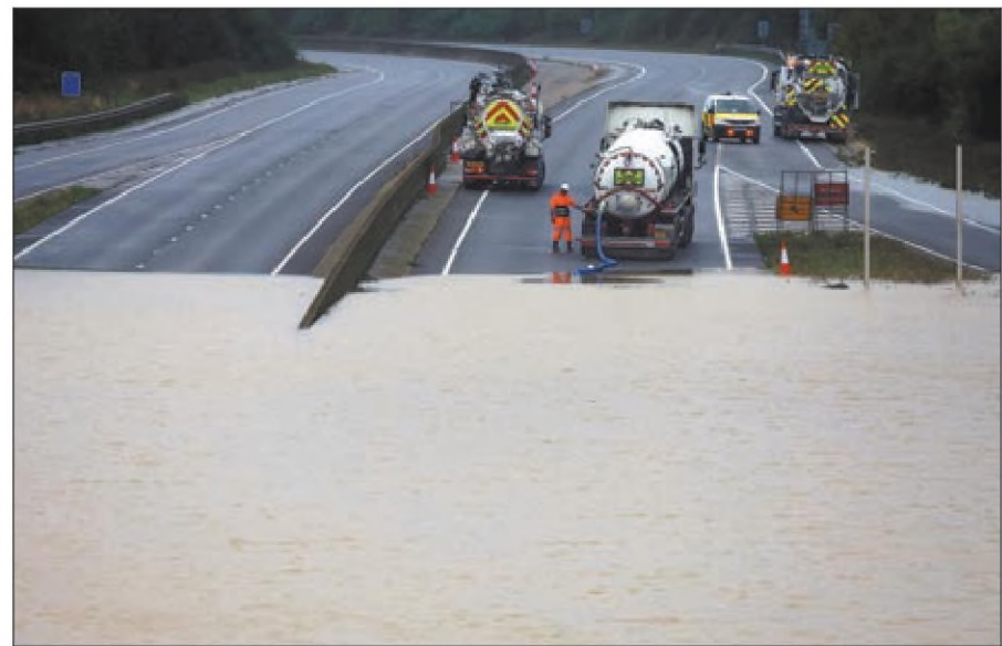
Emergency crews pump floodwaters from a submerged road at Marston Moretaine near Bedford, England, on Monday, after torrential rains lashed parts of England and Wales, disrupting travel and causing significant damage to properties. TOBY MELVILLE / REUTERS
