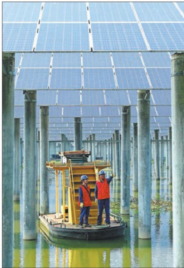
Electricians inspect a lake-based photovoltaic array in Chuzhou, Anhui province, last month. SONG WEIXING / FOR CHINA DAILY
