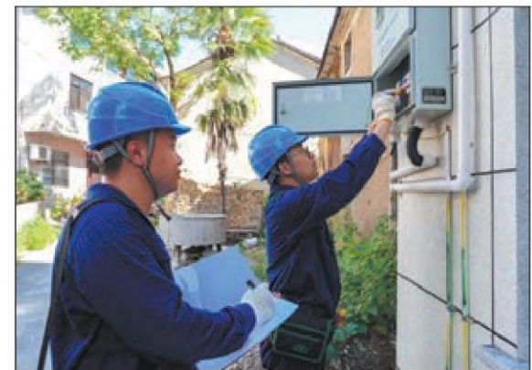
Staff from State Grid Hangzhou Power Supply Co install primary and secondary integrated circuit breakers at low-voltage distributed photovoltaic grid connection points in their service area over the weekend. The breakers provide a safer and more flexible distributed power source for the new power system.
