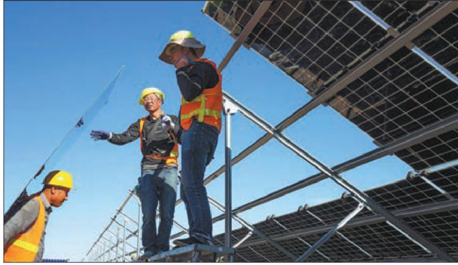
Employees install solar panels at a power station in Zhangye, Gansu province, on Sept. 7. YANG XIAO / FOR CHINA DAILY
