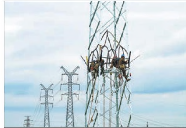
State Grid employees inspect a transmission tower in Taizhou, Jiangsu province, in September. TANG DEHONG / FOR CHINA DAILY
