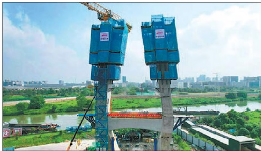
A drone image shows the construction site of a railway bridge along the Yuhang-Deqing Railway in Zhejiang province. Builders of China Railway 24th Bureau Group Corp continued work on the bridge during the weeklong National Day holiday to ensure progress, as the project will play a key role in linking Yuhang district in Hangzhou and Deqing county in Huzhou and boost integrated development within the Yangtze River Delta region. PROVIDED TO CHINA DAILY
