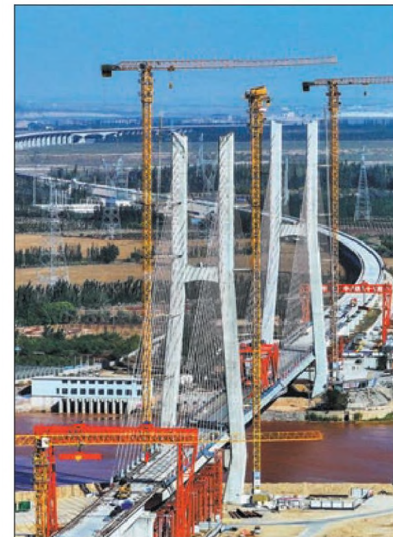
Marking a significant progress in the construction of Baotou-Yinchuan high-speed railway, the final segment of a key bridge over the Yellow River in Wuhai, Inner Mongolia autonomous region, is connected on Wednesday. Designed for a speed of 250 kilometers per hour, the railway will serve as a major transportation artery linking the country's northwest region with the north and northeast region. LIAN ZHEN / XINHUA
