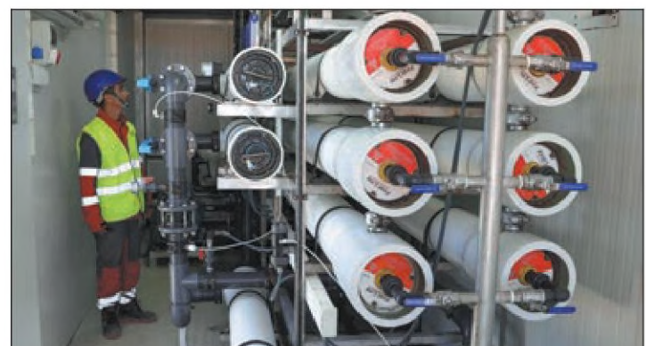
A technician checks on equipment inside a desalination station in Beddouza, Morocco, on July 23. AFP
