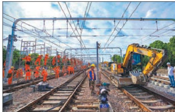
Builders from China Railway No 4 Engineering Group Co Ltd, working on the western extension of Shanghai metro line 13, make a curved section at Beidi Road parking garage into straight tracks to enhance the line's safety and efficiency for trains. ZHAO YUANKUN / FOR CHINA DAILY
