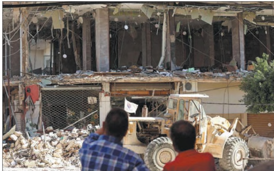
People look at a damaged building after Israeli airstrikes in Tyre, Lebanon, on Monday. AZIZ TAHER / REUTERS
