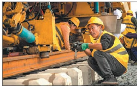
CREC4 employees lay tracks on the Chongzuo-Pingxiang high-speed railway in the Guangxi Zhuang autonomous region on Monday. ZHAO MENGTING / FOR CHINA DAILY
