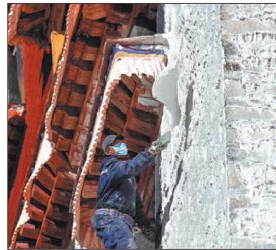
A worker splashes paint on the exterior wall of the Potala Palace in Lhasa, Xizang autonomous region, on Monday. The annual beautification of the palace not only serves an aesthetic purpose but also plays a crucial role in protecting the structure.
