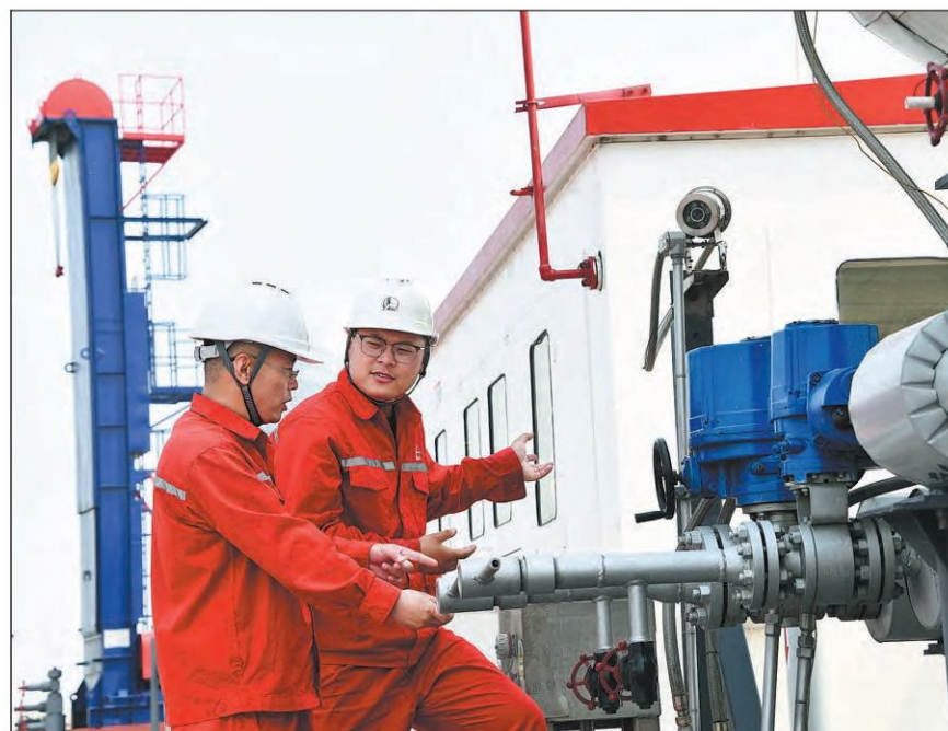
Sinopec employees check CCUS equipment operations in Dongying, Shandong province. FAN CHANGGUO / XINHUA
