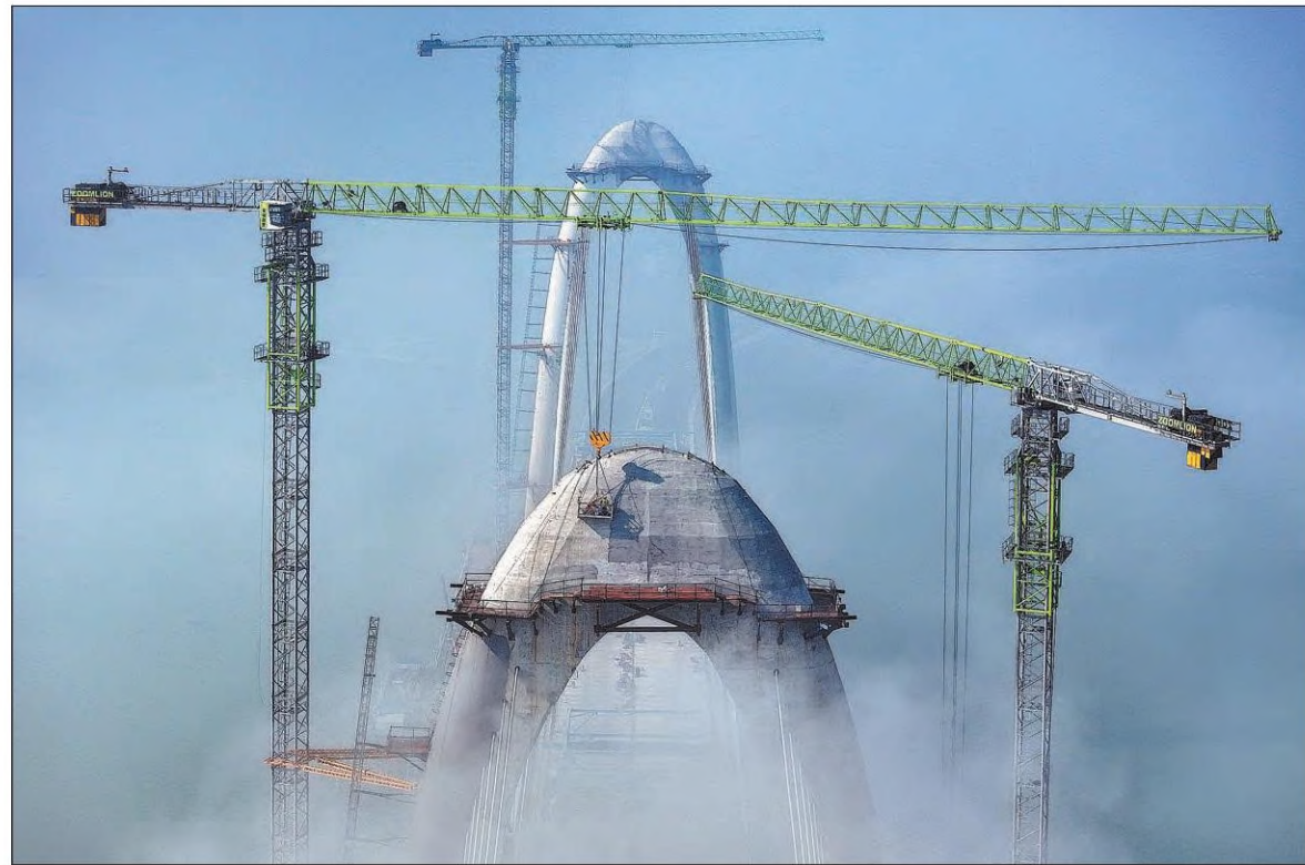
The main bridge of the Xinglian Road Grand Link across the Xiangjiang River is under construction in Changsha, Hunan province, on Wednesday. The bridge will be nearly 5 kilometers long upon completion, making it the longest bridge in the provincial capital.
