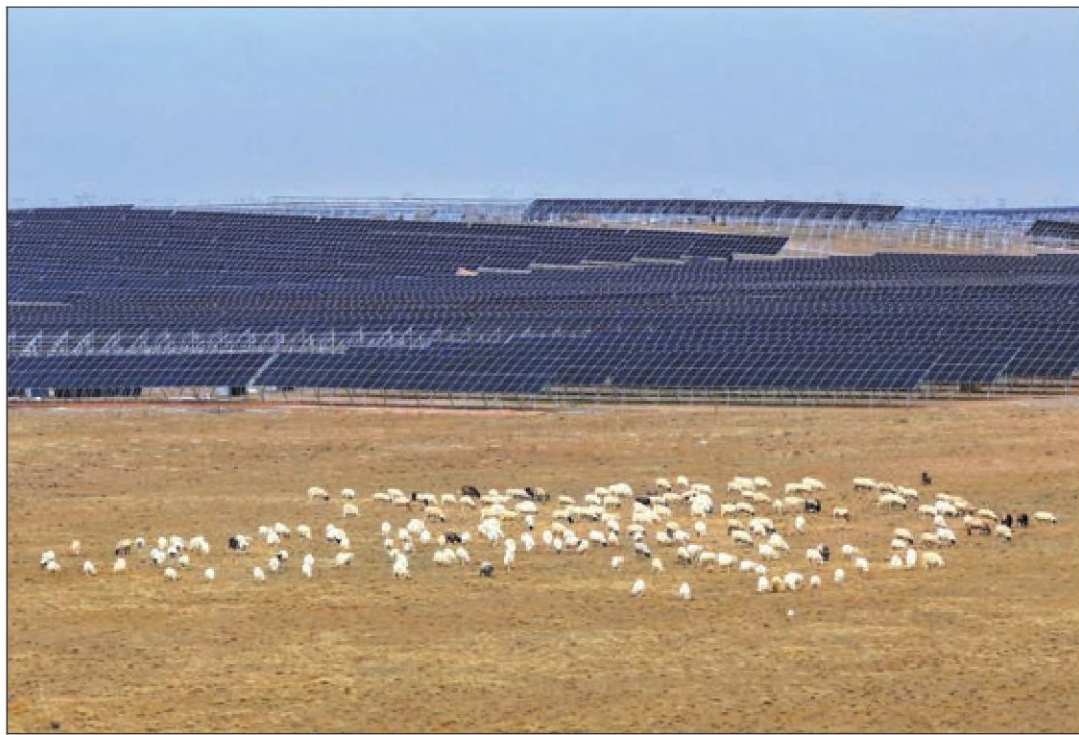
A photovoltaic power generation plant sprawls across the grassland in Otog Front Banner in Ordos, Inner Mongolia autonomous region, in November last year. WANG ZHENG / XINHUA
