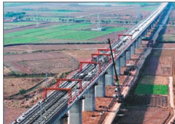
A drone image shows the construction site of the Wuhan-Yichang section of the Shanghai-Chongqing-Chengdu high-speed railway in Hubei province. The 313-kilometer section, which is being built by the 24th bureau of State-owned infrastructure builder China Railway Construction Corp as a critical part of the national major horizontal rail network, has had its ballastless track completed — another major milestone ahead of its expected operation next year. PROVIDED TO CHINA DAILY
