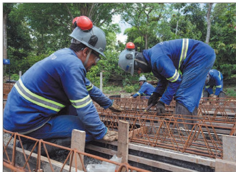
Brazilian workers are seen at the construction site of the West-East Integration Railway Project in Bahia state, Brazil, on Feb 6. China Railway No 10 Engineering Co also participated in the project. WANG TIANCONG / XINHUA
