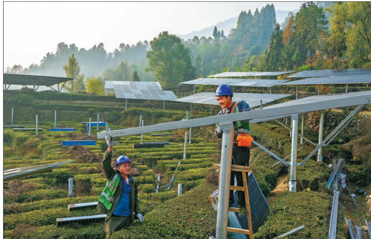
Technicians install solar photovoltaic panels at a power station in Zigui county, Hubei province, in November. ZHENG JIAYU / FOR CHINA DAILY
