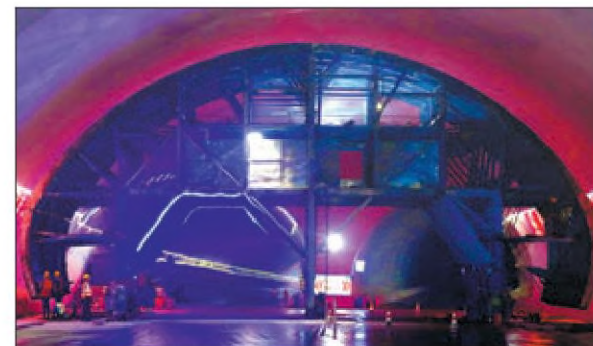
Staffers from CREC4 Seventh Engineering work on the Jiaozhou Bay Second Tunnel in Qingdao, Shandong province. LI PINGHUI / FOR CHINA DAILY
