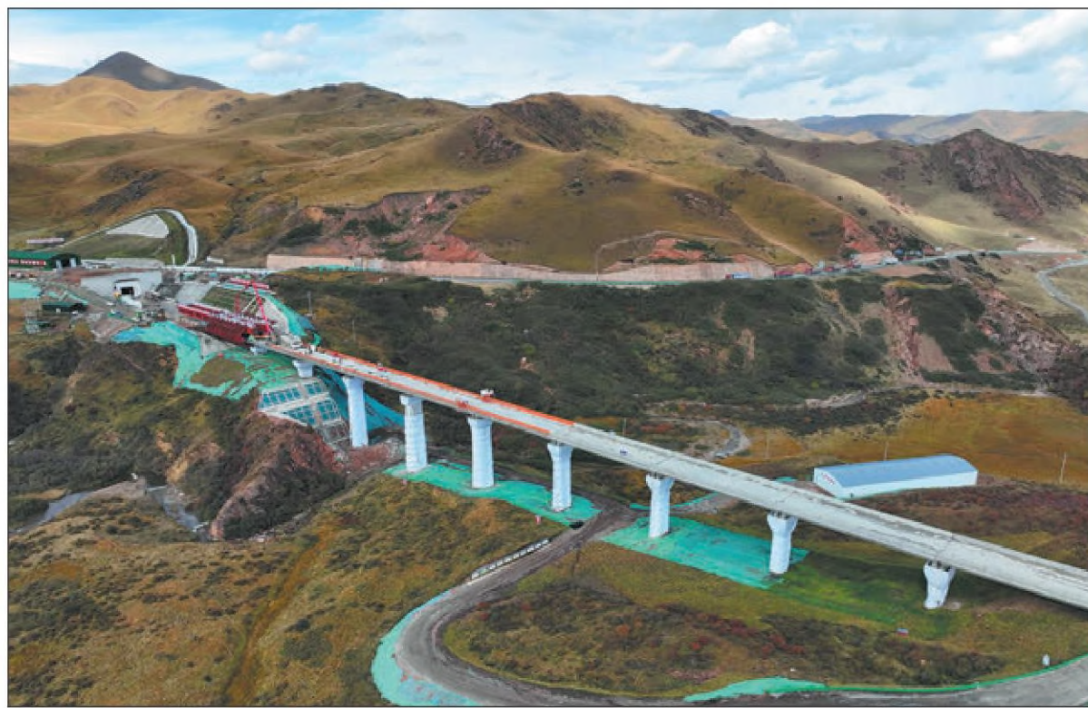
Builders from China Railway No 4 Engineering Group Co Ltd make progress in building the Xining-Chengdu railway. XING JIANG / FOR CHINA DAILY
