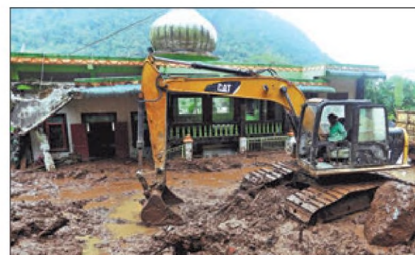
An excavator moves soil during a search and rescue operation at the site of a landslide in a village in Karo, North Sumatra Province, Indonesia, on Monday. REUTERS
