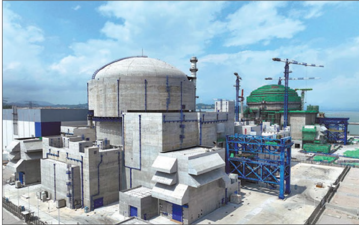
A photograph taken in September shows the construction site of a nuclear power plant in Zhangzhou, Fujian province. LIN SHANCHUAN / XINHUA
