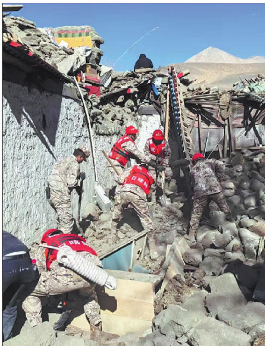
Rescue efforts underway on Tuesday at an earthquake-affected area in Dingri county of Shigatse, Southwest China's Xizang autonomous region. The magnitude 6.8 quake brought down scores of buildings, killing at least 126 people and injuring 188 others. There are 27 villages and approximately 6,900 people living within a 20-kilometer radius of the earthquake's epicenter. LIU YOUSHEG / XINHUA
