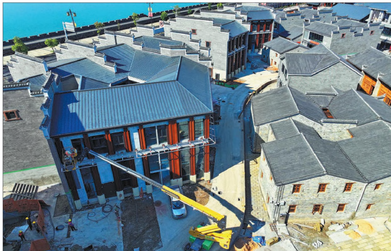
Workers renovate a house in Ji'an, Jiangxi province, in November. ZHU HAIPENG / FOR CHINA DAILY
