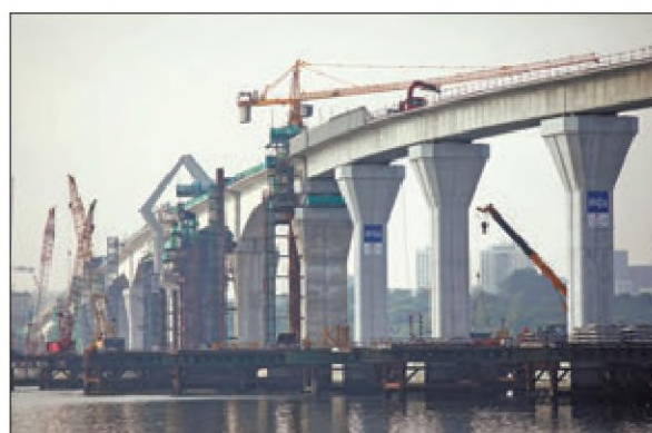
The Johor Bahru-Singapore Rapid Transit System Link is under construction in Johor Bahru, Malaysia, on Sept. 23. SAMSUL SAID VIA GETTY IMAGES
