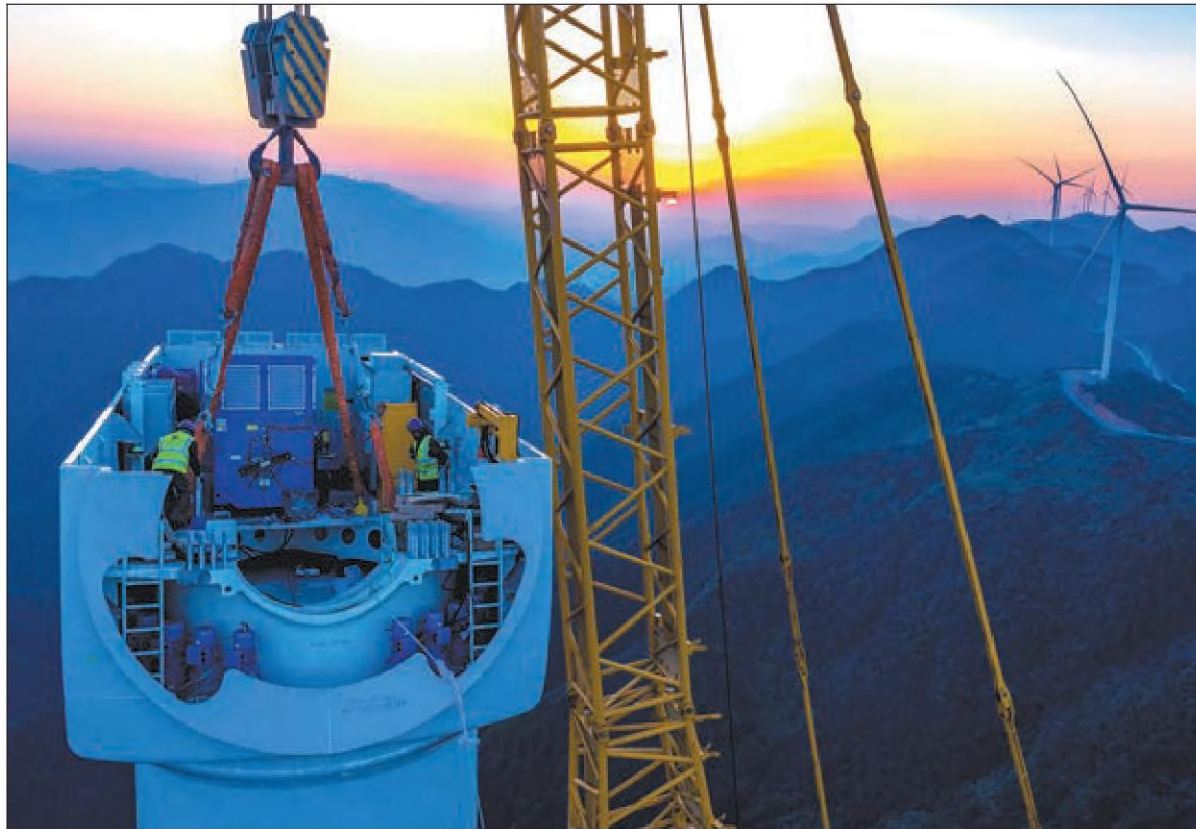
Workers install wind turbines at a wind farm project construction site in Ruichang, Jiangxi province, on Dec 19. WEI DONGSHENG / FOR CHINA DAILY
