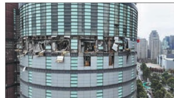
The damaged facade of a department store in the city of Taichung in central Taiwan is seen on Thursday after a gas explosion on the premises killed four people and injured 26. YUFU LIAO / AFP
