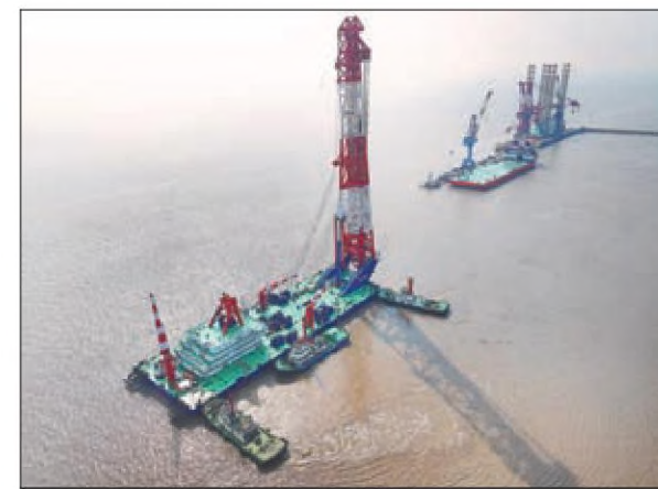
Erhang Changqing, the world's largest pile-driving vessel, departs Qidong, Jiangsu province, on Monday, en route to build the Hangzhou Bay Cross-Sea Railway Bridge. XU CONGJUN / FOR CHINA DAILY
