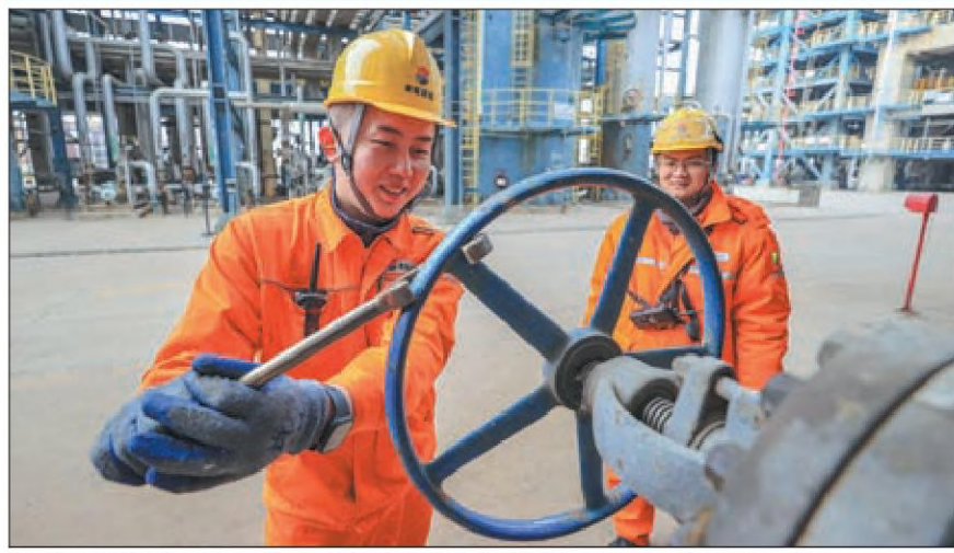
Employees check equipment at a petrochemical plant in Lianyungang, Jiangsu province. SI WEI / FOR CHINA DAILY
