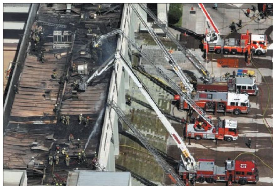
Firefighters try to douse the flames at the central building of a police academy in Santiago, Chile, on Wednesday. The fire affected the third floor of the building as 18 engines and more than 150 volunteer firefighters were dispatched to fight the blaze. JAVIER TORRES / AFP
