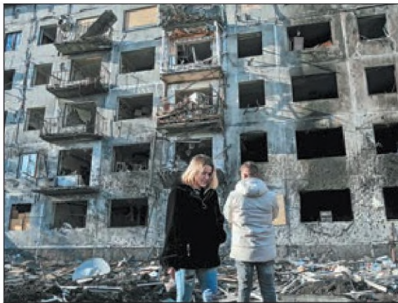
People look at a damaged building two days after Russian shelling in Donetsk, on Sunday. MARIA SENOVILLA / EPA-EFE
