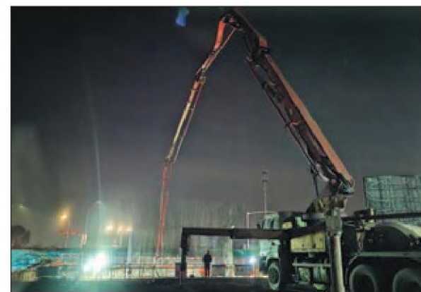
A construction worker from China Railway 24th Bureau Group monitors a crane in the middle of cement pouring for the concrete base of the Tenglong Avenue bridge in Changzhou, Jiangsu province, on Friday. The project will serve as a vital thoroughfare in Changzhou, and is designed to enhance connections between its south and north regions while promoting integrated development. PROVIDED TO CHINA DAILY
