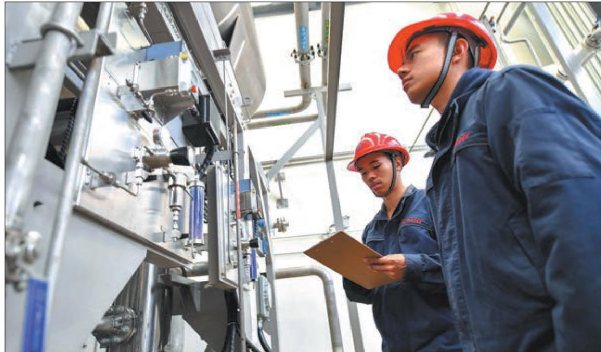
Workers inspect equipment at a station that produces hydrogen and charges hydrogen-powered vehicles in Changsha, Hunan province, in March last year. The station is able to serve more than 100 vehicles a day with clean, green energy. CHEN ZEGUO / XINHUA
