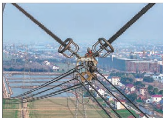
A technician conducts maintenance work on a high-voltage power line in Nantong, Jiangsu province, on Feb 27.
