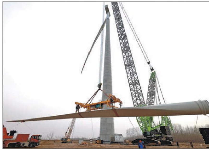
An image shows the installation of a wind turbine blade at a wind farm in Xingtai, Hebei province, on March 12. WANG LEI / FOR CHINA DAILY
