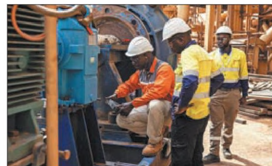
Workers fix a water pump inside the Eramet floating wet concentration plant in Lompoul, Senegal, on Feb 12.
