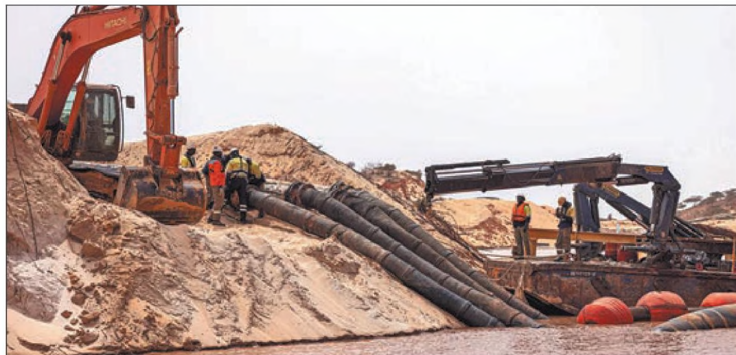
Workers adjust dredging pipes at Eramet's floating wet concentration plant in Lompoul, Senegal, on Feb 12.
