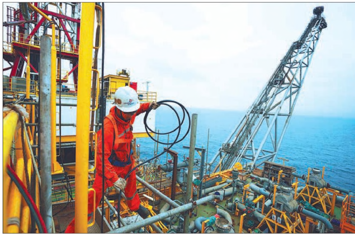
An engineer works at the Dongfang 13-2 gas fields project, China's largest offshore high-temperature and high-pressure gas fields project, located offshore near Dongfang, Hainan province. YUAN CHEN / FOR CHINA DAILY
