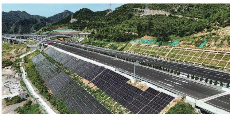
Photovoltaic panels installed along the Jinan-Weifang expressway in Shandong province. PROVIDED TO CHINA DAILY
