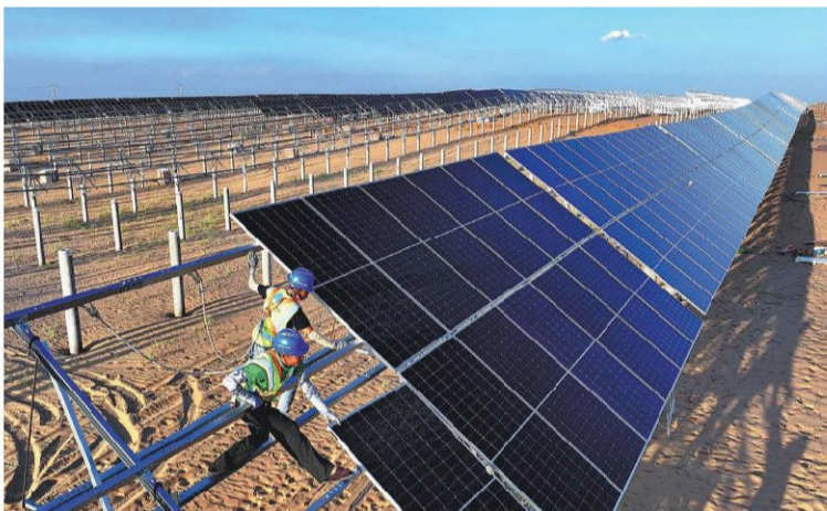
Workers install photovoltaic panels at a new energy base in the Kubuqi Desert in Ordos. PROVIDED TO CHINA DAILY
