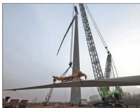
Workers install a wind turbine blade in Xingtai, Hebei province. WANG LEI / FOR CHINA DAILY
