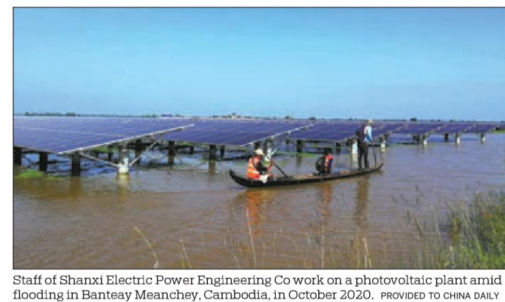
Staff of Shanxi Electric Power Engineering Co work on a photovoltaic plant amid flooding in Banteay Meanchey, Cambodia, in October 2020. PROVIDED TO CHINA DAILY
