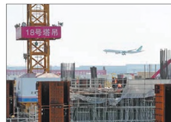
An aerial view of the construction site of Shanghai East Railway Station. GAO ERQIANG / CHINA DAILY
