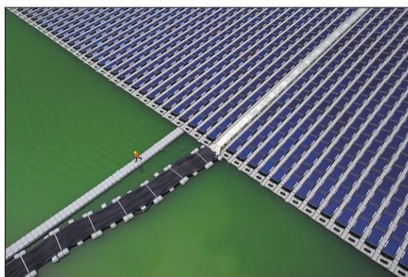
Top: Joggers pass by a floating solar panel farm on the Bedok Reservoir in Singapore in 2023. DAVID GOLDMAN / AP. Above: Workers walk across a floating solar panel farm in Binh Thuan Province, Vietnam, in 2021. NGUYEN TAN TUAN / SOLENT NEWS
