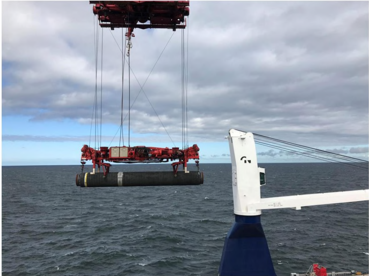
Allseas' deep sea pipe laying ship Solitaire lays a pipe for Nord Stream 2 pipeline in the Baltic Sea September 13, 2019. REUTERS/Stine Jacobsen/File Photo
