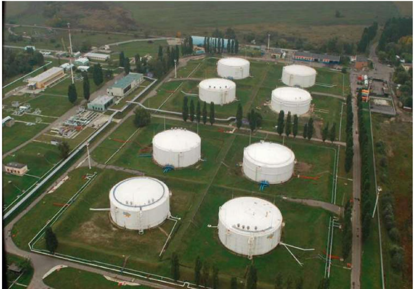
A gas storage facility from Ukraine's state gas operator Naftogaz. Photo: Naftogaz
