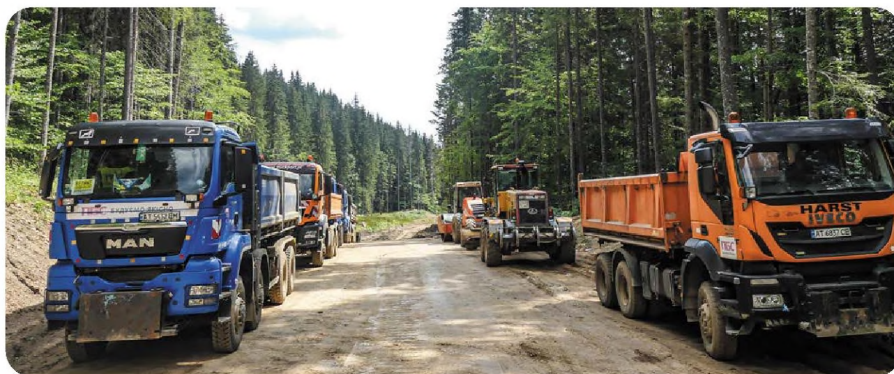
New “forest highway” under construction on 22.08.2023, two weeks before the contract with PBS was signed
